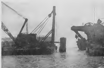
As Finger Pier No. 1 nears completion, these barges finish their work of clearing away the east end of the T dock. Here the last group of pilings is removed. It is expected that by the middle of December work will begin on Finger Pier No. 2.
